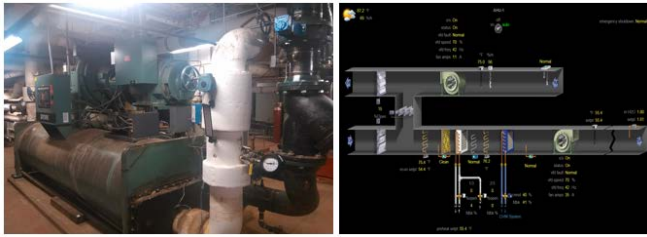
Figure 5 Chiller and BAS connected to the HVAC system
