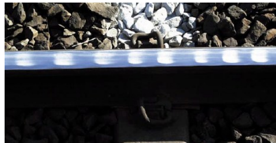
Figure 3. Rail corrugation (Rail defects, 2002).
