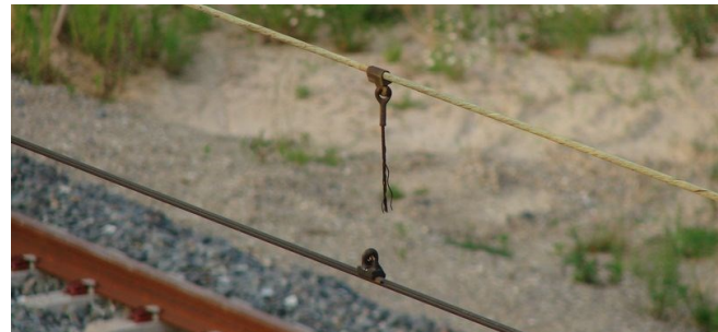
Figure 4. Dropper failure caused by fatigue.
